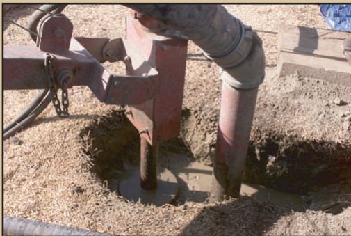
The pickup pump "vacuums" mud and cuttings from the borehole and diverts them to the shaker or mud-filtering system.
